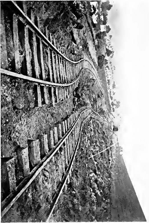
A. Earth-slump north of Tomales, carrying railway roadbed with it. Track was straight before earthquake. R. S. H.
